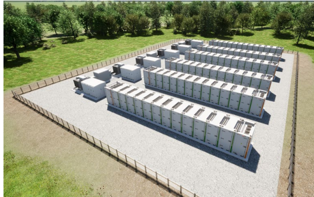
Battery Storage Compound
