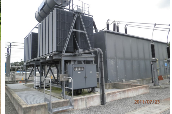
400 kV Power Transformer
